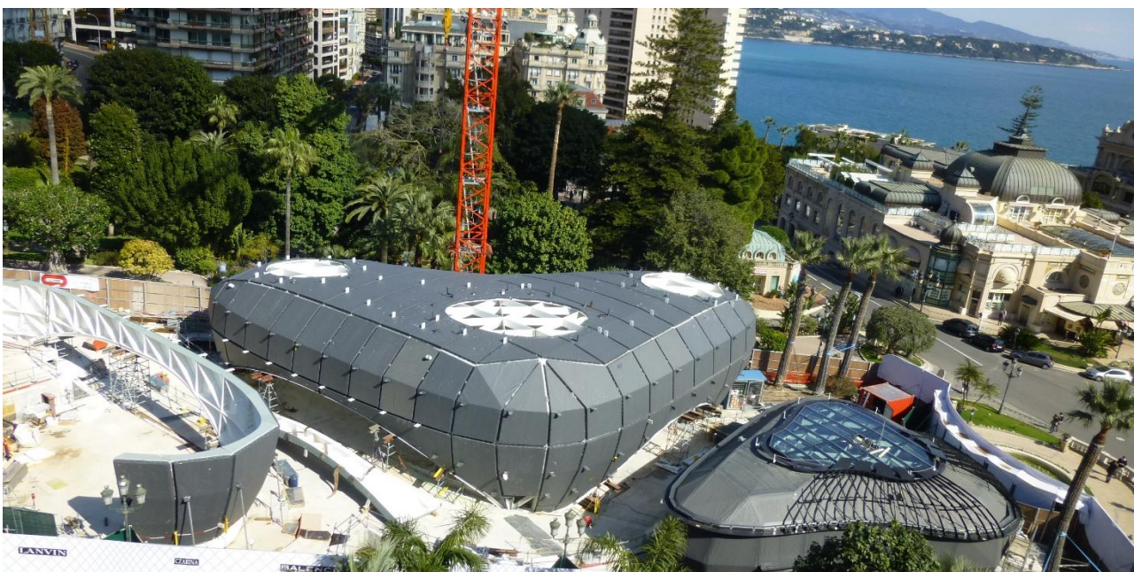
Figure 6: Weathering panel shell system and secondary structure during installation off site work.
